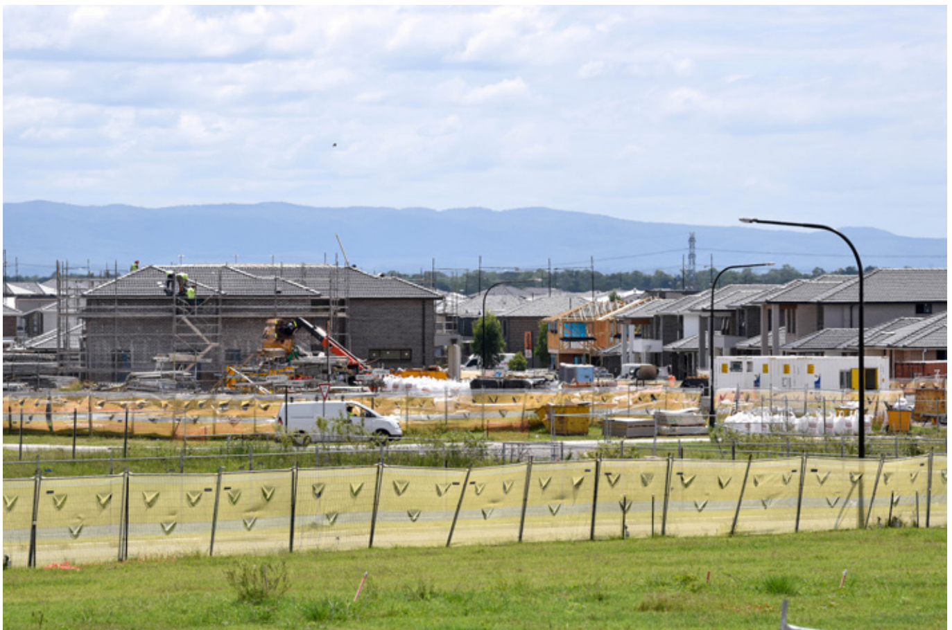
New housing being constructed at Marsden Park, looking towards the Blue Mountains.
