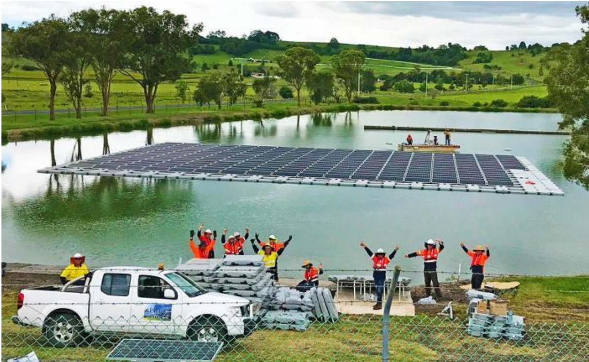
FIGURE 14: LISMORE CITY COUNCIL'S 'FARMING THE SUN' FLOATING SOLAR ARRAY ON EAST LISMORE STP
